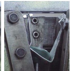
Detail following lug breakage.
