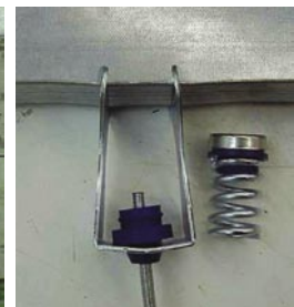
Detail following breakage.
